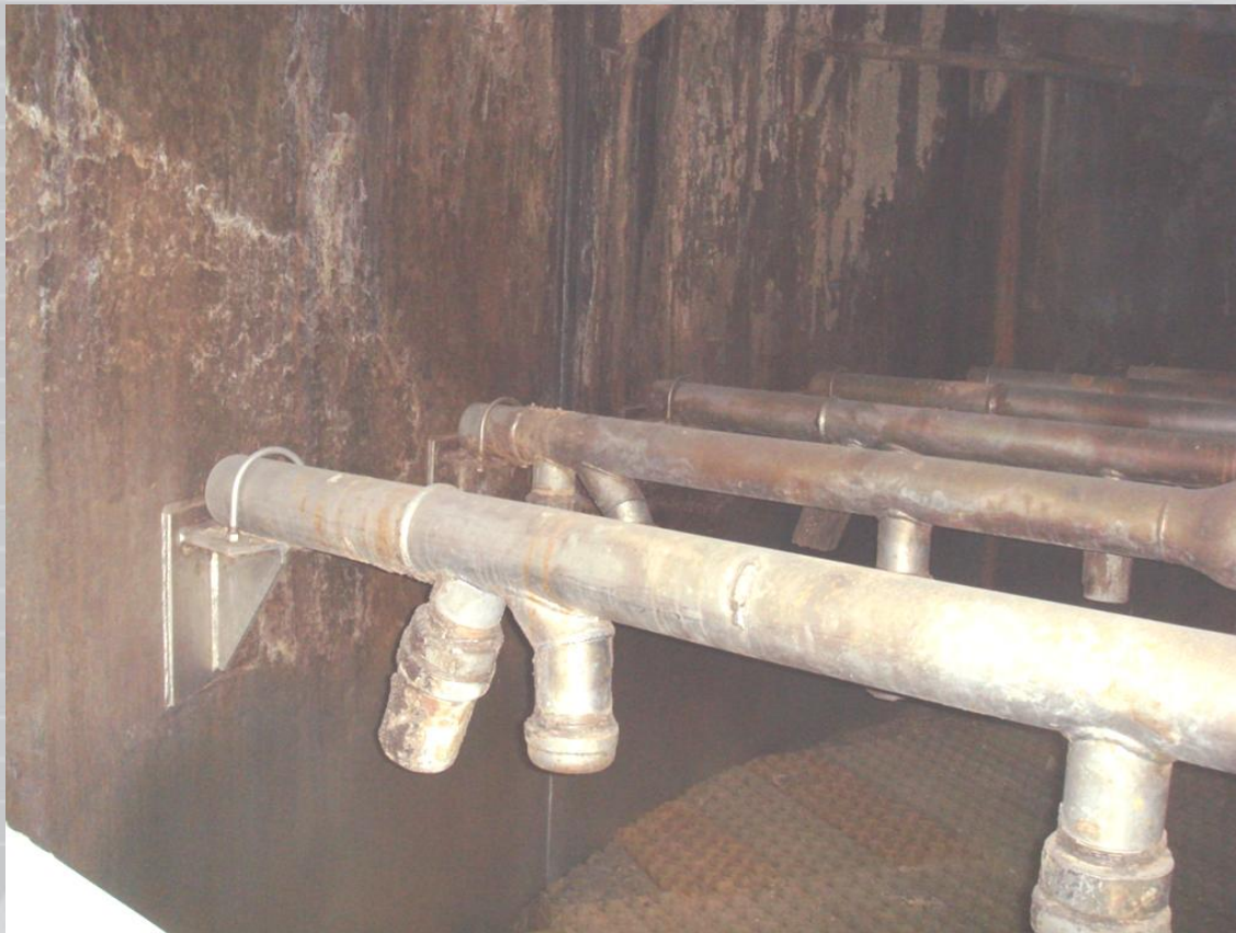
Nozzles next to the wall
