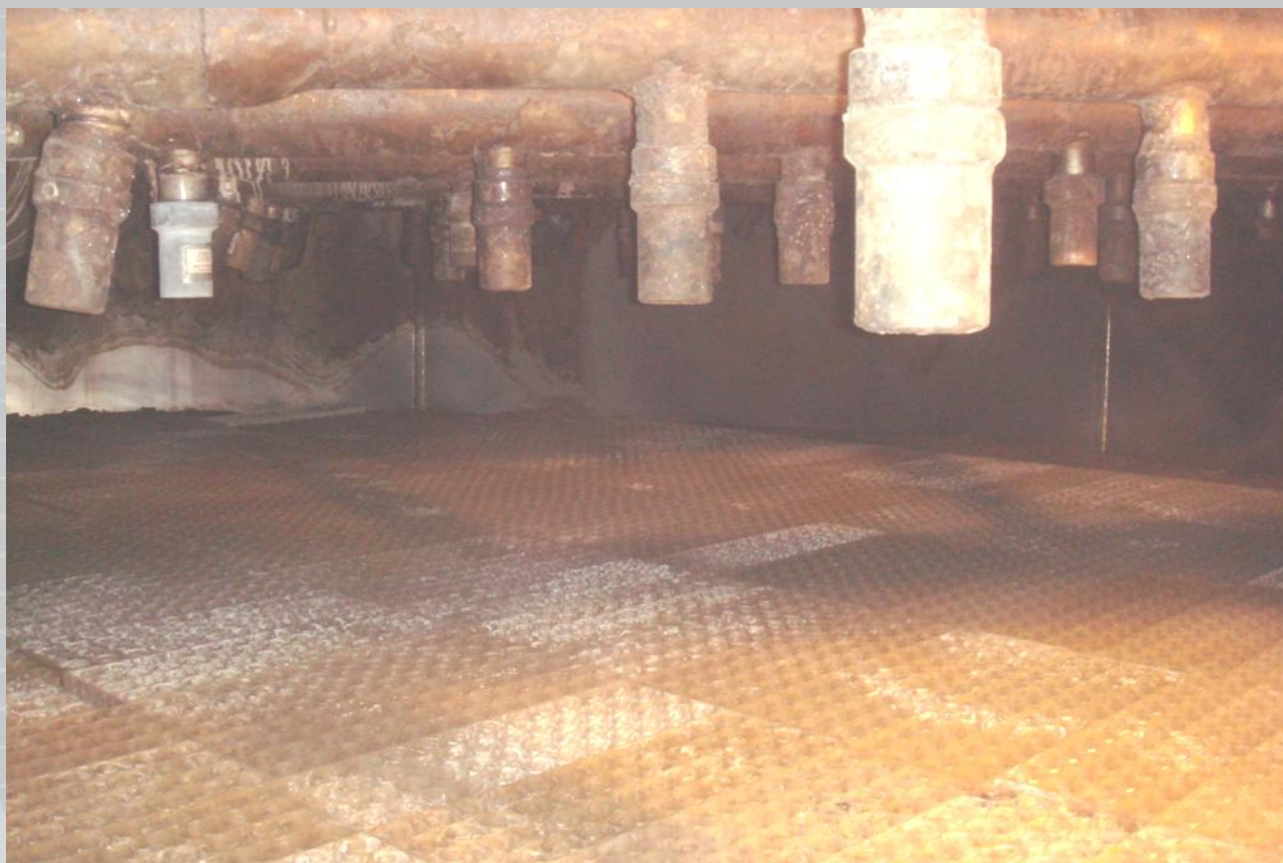
Fullcone Nozzles above WFC
